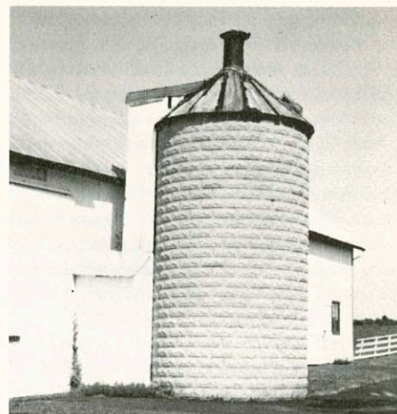
A beautiful concrete block silo. Joseph Baumgart farm north of Mishicot. Popular in northern part of county.
